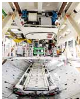
Crammed full of technology – a view of the front part of the Herrenknecht TBM.
