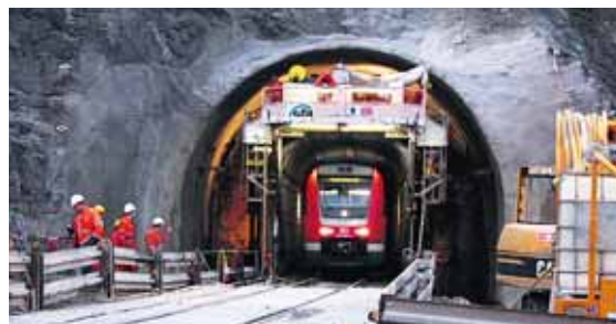
Using this new method, work on tunnels can now be carried out with trains running.
