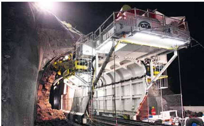
The machine developed for the tunnel-in-a-tunnel principle was also used for the renovation of the Jähröder Tunnel in Rhineland-Palatinate. Photos: DB ProjektBau GmbH/Matthias Oettel
