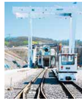
View of the TBM and the railway tracks used for removal of soil and rock. Photos: DB AG/Ralf Kranert
